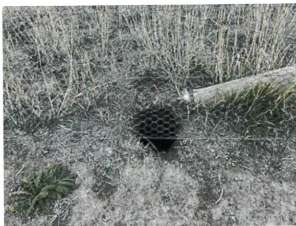
Photo 5: Hole made during fence construction that was not filled in
